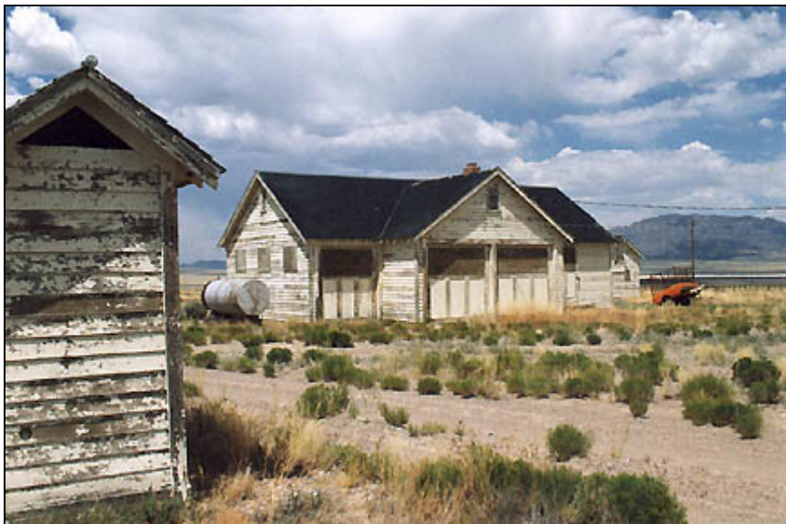
Peeling paint and boarded up DRES buildings. July 17, 2005 photograph © by Linda Moulton Howe.
